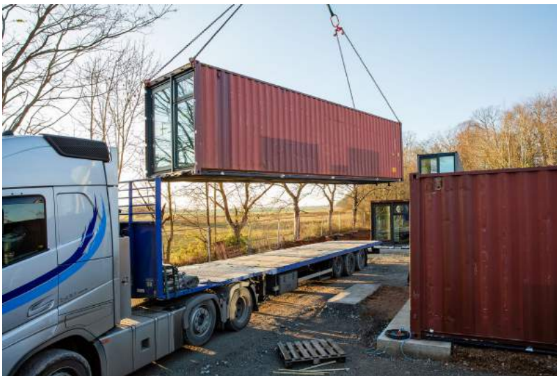
The fully finished containers were delivered using normal site logistics with the entire group in place after four days of onsite assembly.
